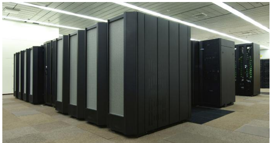
ECMWF's current High Performance Computing Facility (HPCF). One of the most powerful in Europe, comprises two identical independent IBM Cluster 1600 supercomputers based on POWER5 processor technology.
