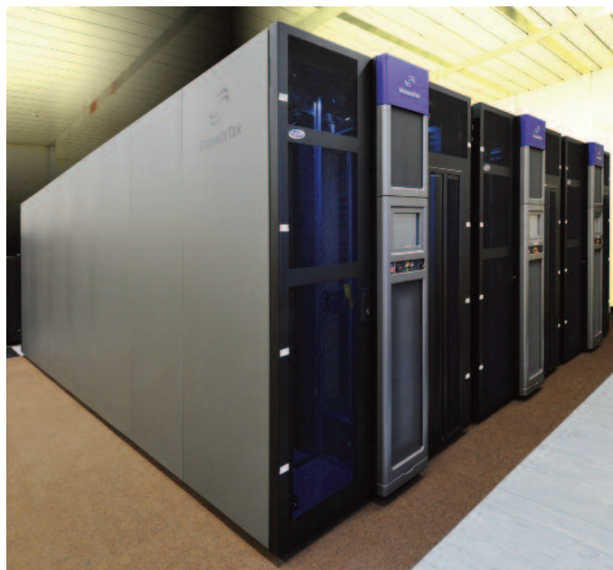
New automated tape library. The automated tape library is part of ECMWF's data handling system. The new library will allow a large number of concurrent retrieval requests and very high tape exchange rates.
