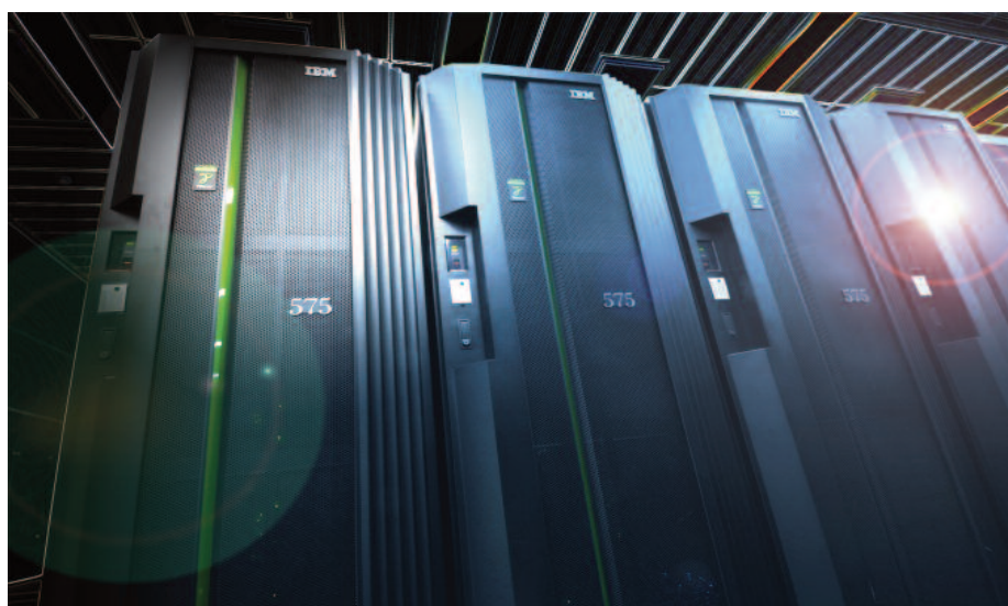
Part of ECMWF's high-performance computing facility (HPCF). The HPCF consists of two identical, independent IBM Cluster 1600 supercomputers and storage clusters.
